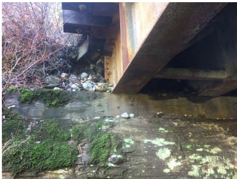
Left bank ballast wall has failed
