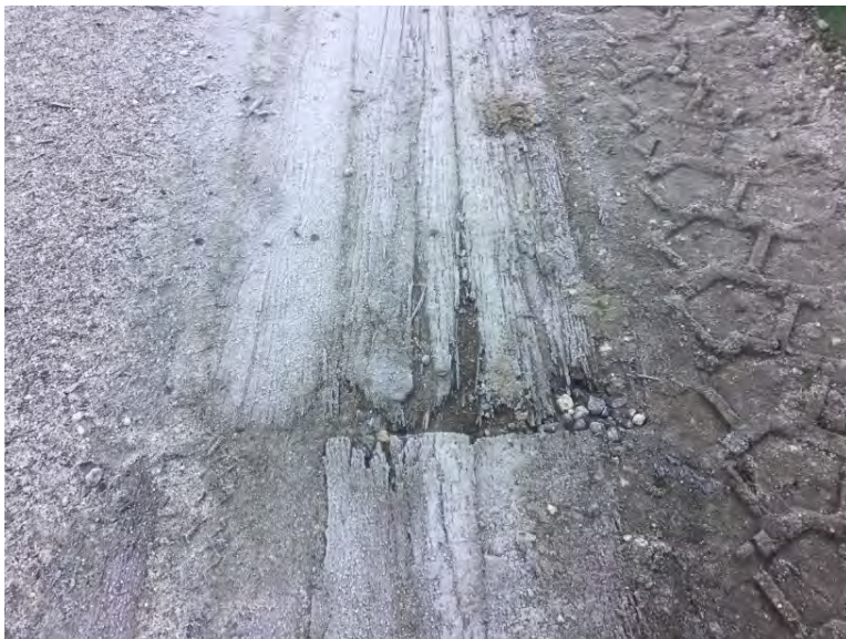
Deck plank condition
