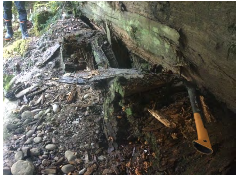
Mudsills at right bank in overall poor condition
