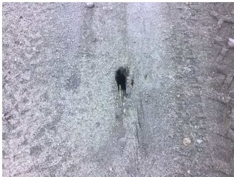
Holes in deck
