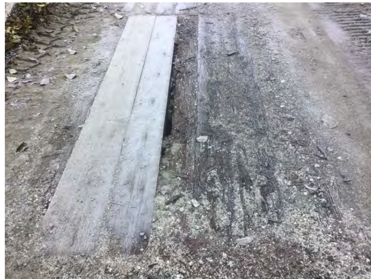
Deck plank condition
